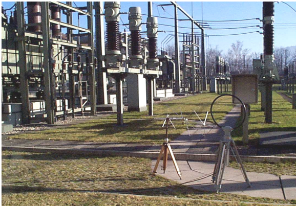
Field strength measurement at a transformer substation in Freiburg
